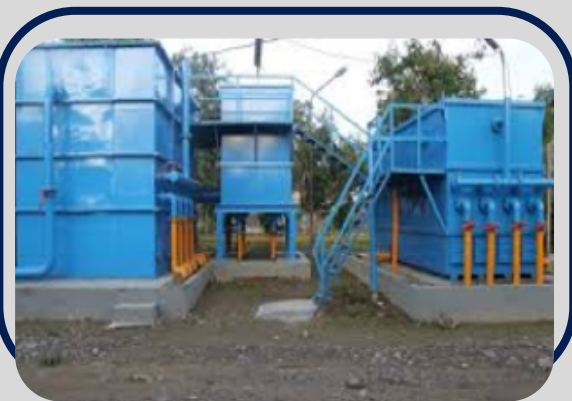
4. Water Treatment Plant
